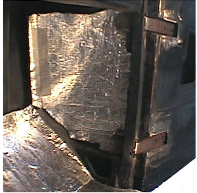
Cowl Absorber Panel ready to tape.
