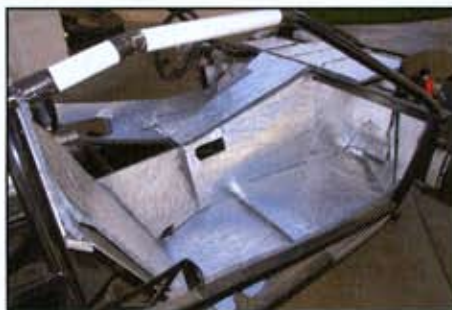
Note how thoroughly the material will cover every surface in the cockpit, and in every nook and cranny. The foil-backed insulation is still being dry-fitted at this stage.
