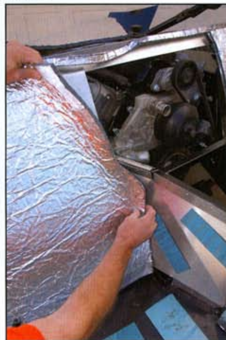
Next dry-fit the pre-cut piece of foil-backed insulation in place, making sure it follows any curves or corners. Note how close the mid-mounted engine is to the back of the cockpit. Adding shielding for both heat and sound is obviously a benefit for driver and passenger comfort. (pipe). So reducing noise levels starts with minimizing vibration, like placing your hand on the skin of a drum.
