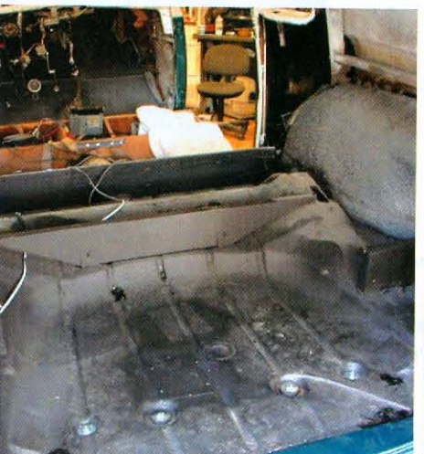
11) Looking in the back door, with the wood floor removed, we find plenty of heat- and sound-generating surfaces the factory had left completely bare.
