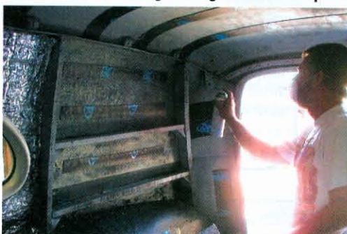
23) With all the pieces cut to fit each position, Cox begins the sidewall installation. Here, he's using the supplied spray can to apply an even coat of adhesive to the area. Note the fume-filtering facemask.
