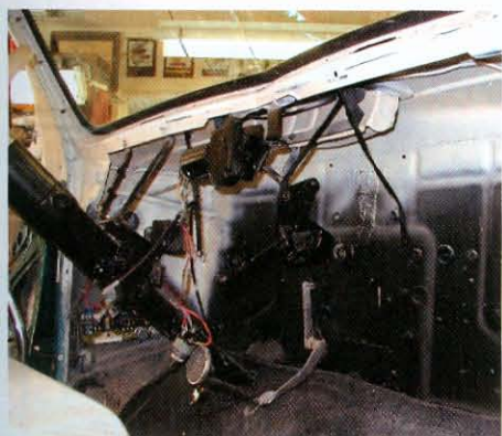
5) Here's the firewall after complete removal of the original insulator. We painted the light color to facilitate photography. The original mounting holes along the top will be reused to mount the new insulator. Note all the pressed-in reinforcements. These eliminate the need for the vibration-killing sound-insulation strips.
