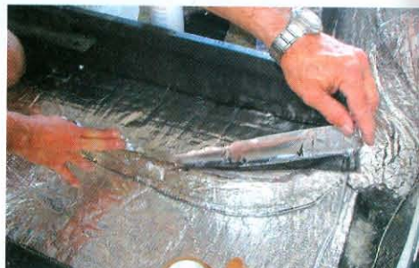
27) After all the insulation is glued in place, it's time to seal every joint and seam with the supplied foil tape. This forms a one-piece inner skin of insulation with no small cracks or holes to allow heat to penetrate.
