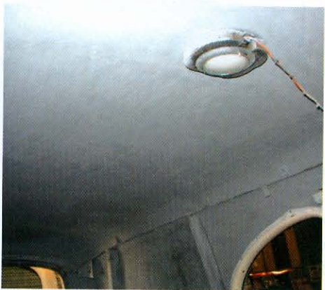
10) The bare sheetmetal roof and walls were cleaned with a power wire brush and then thoroughly washed with hot, soapy water, rinsed and blown dry with the air hose. We then rattle-canned on a coat of light-gray primer to prevent surface rust and as a photographic aid.
