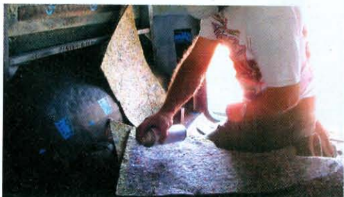
24) Next comes a very important step: spraying a matching, even coat of adhesive on the insulation piece. We're sure you've noticed that the insulation sheets are installed foil side in. This allows the rag side to absorb the heat and the foil side to block it from getting into the interior.
