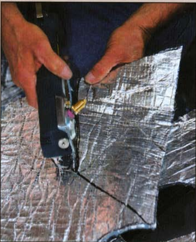
Use a Sharpie pen to outline the areas to be cut. Electric scissors make the job go much faster.
