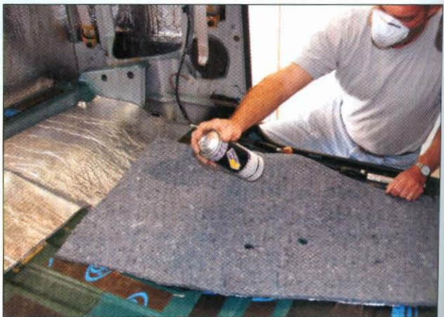
Spray adhesive on the underside of the padding. A double application on the edges is a good idea to ensure a tight bond.
