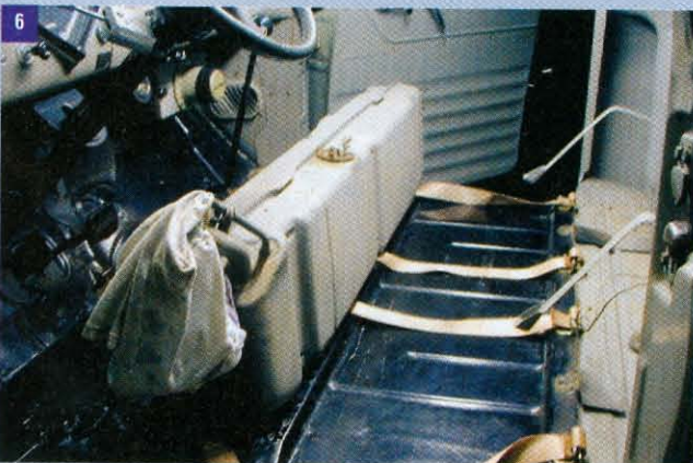
6 We loosened the gas tank and moved it forward to access the cab's rear wall. There was plenty of room to work around it.
